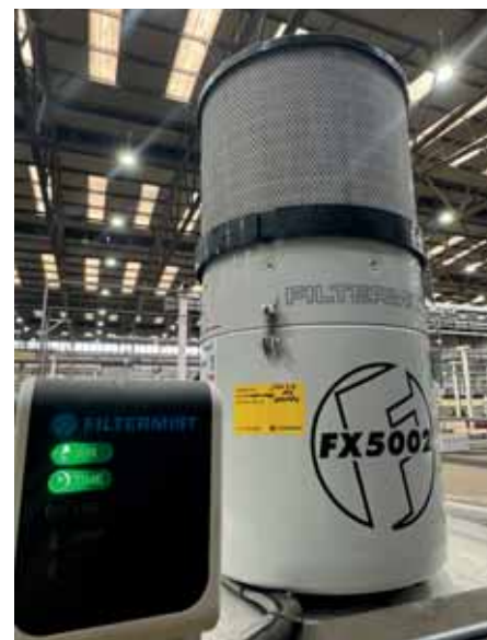
The Filtermist FX5002 system with monitoring at Crittall Windows.
