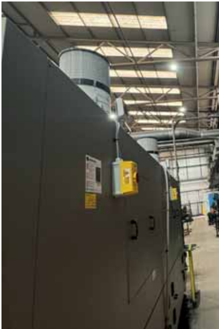
Filtermist extraction systems sitting neatly above the Crittall Windows machine tools.
