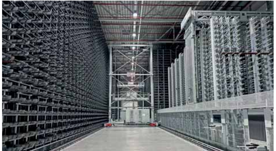
The new storage system at SEW is a combination of a KASTO Unicomcompact honeycomb storage facility with 5,140 cassettes and a KASTOcenter sawing centre with 450 storage locations.
