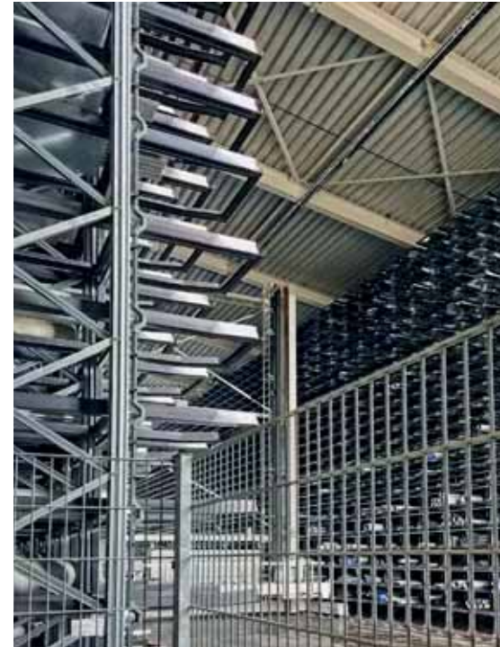
The KASTO Unicomact storage system installed at Austrian tube stockholder Karl Mertl Handelsges significantly increased storage capacity and improved safety.
