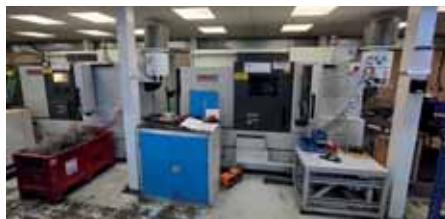
Clarion LEV multiple installations on XYZ machines.
